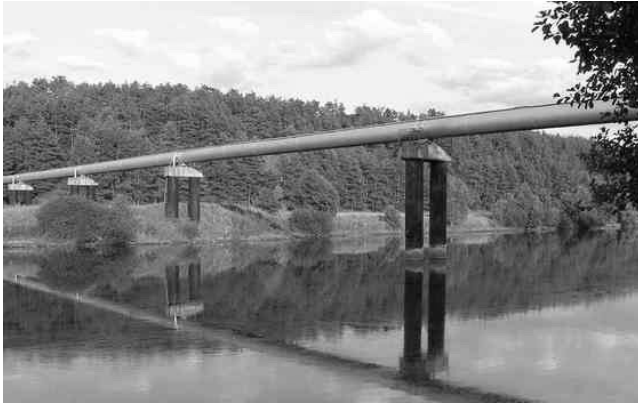
Fig.1. "Union" pipeline air passage (Ukraine)
