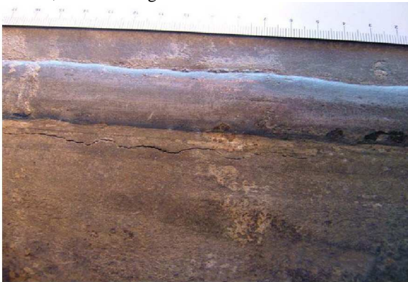
Figure 2 – Longitudinal crack (frontally)
