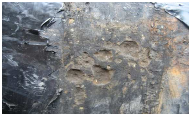
Figure 1 – Corrosion damage to metal pipe
